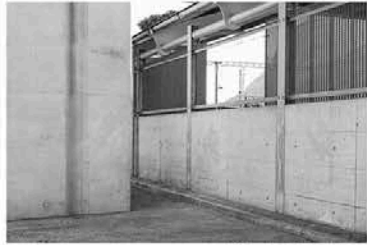
Fig. 9. Exterior view of a building with a concrete wall and a window - Architecture Department, 2023
